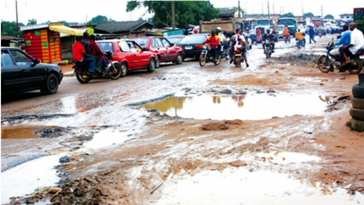
Figure 2: Unmotorable Road, Commonly Sighted in Many University Host Communities in Nigeria
