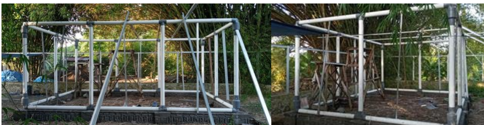
Figure 12: Ring Beam Job Results
