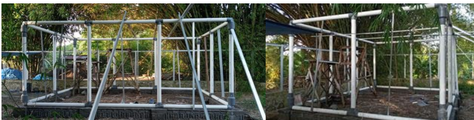
Figure 12: Ring Beam Job Results
